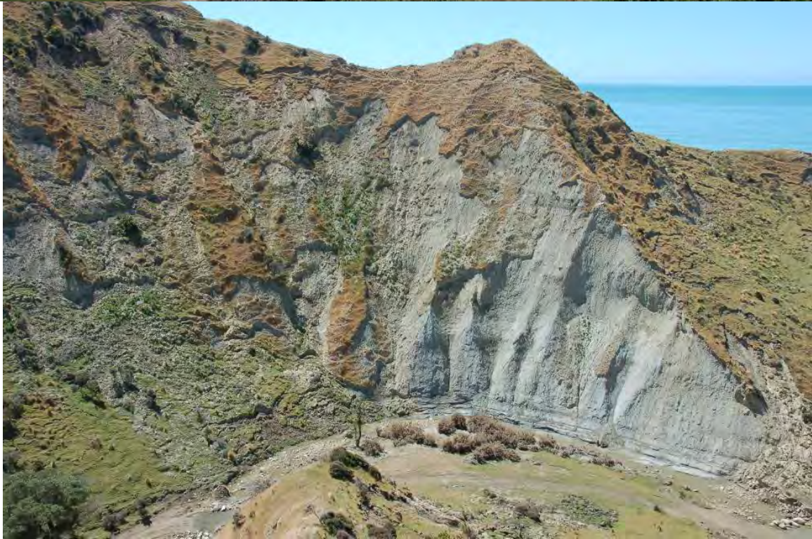
PP9f (top – January 2008, bottom – December 2008) – an historically unstable slope that has been further and severely affected by slipping in lower Kate Valley.
