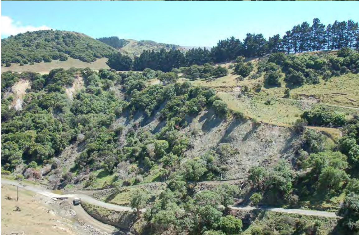
PP9c (top – January 2008, bottom – December 2008) – slips under coastal mixed broadleaved forest removing much of the forest cover.
